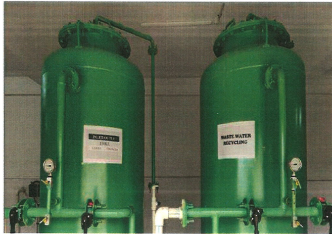
Figure 6. Sewage Treatment Plant
