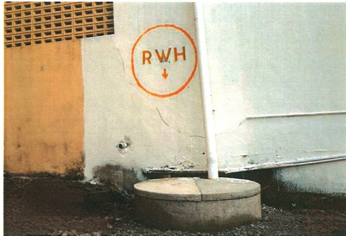
Figure 2: Rain water harvesting system
